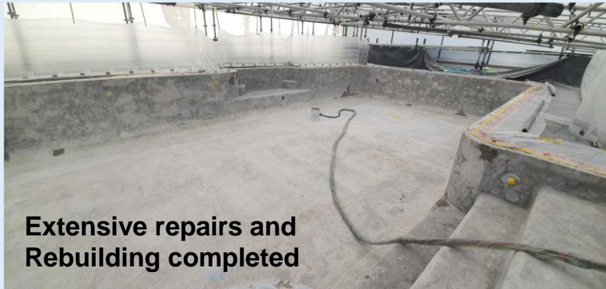
There were many damaged areas to repair
